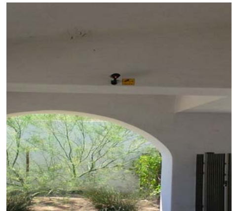
Thanks to a donation from a local business owner, cameras were recently installed at the Mead Valley Community Center.
