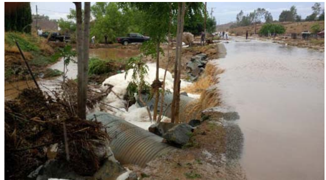
Water pours over Marie St. even after the rain had stopped.
